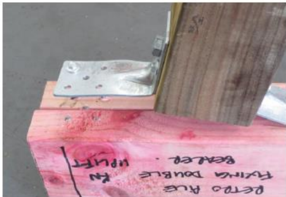
Failure after loading
