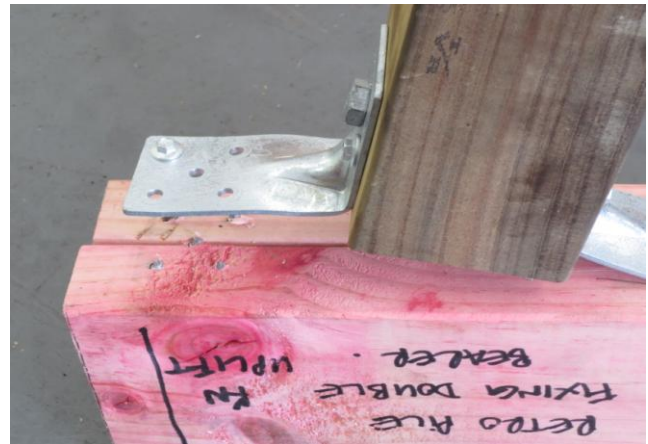
Failure after loading
